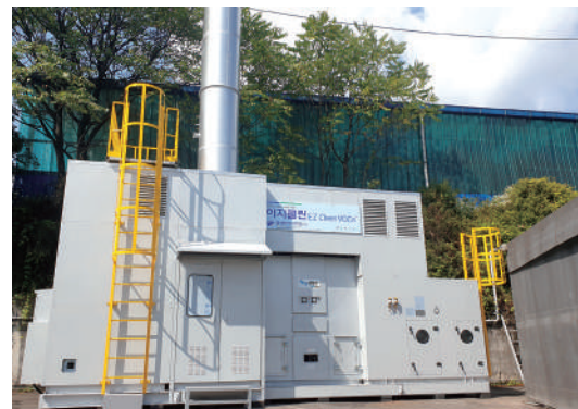
Gaseong Co., Ltd. [EZ Clean 400-125CMM]
